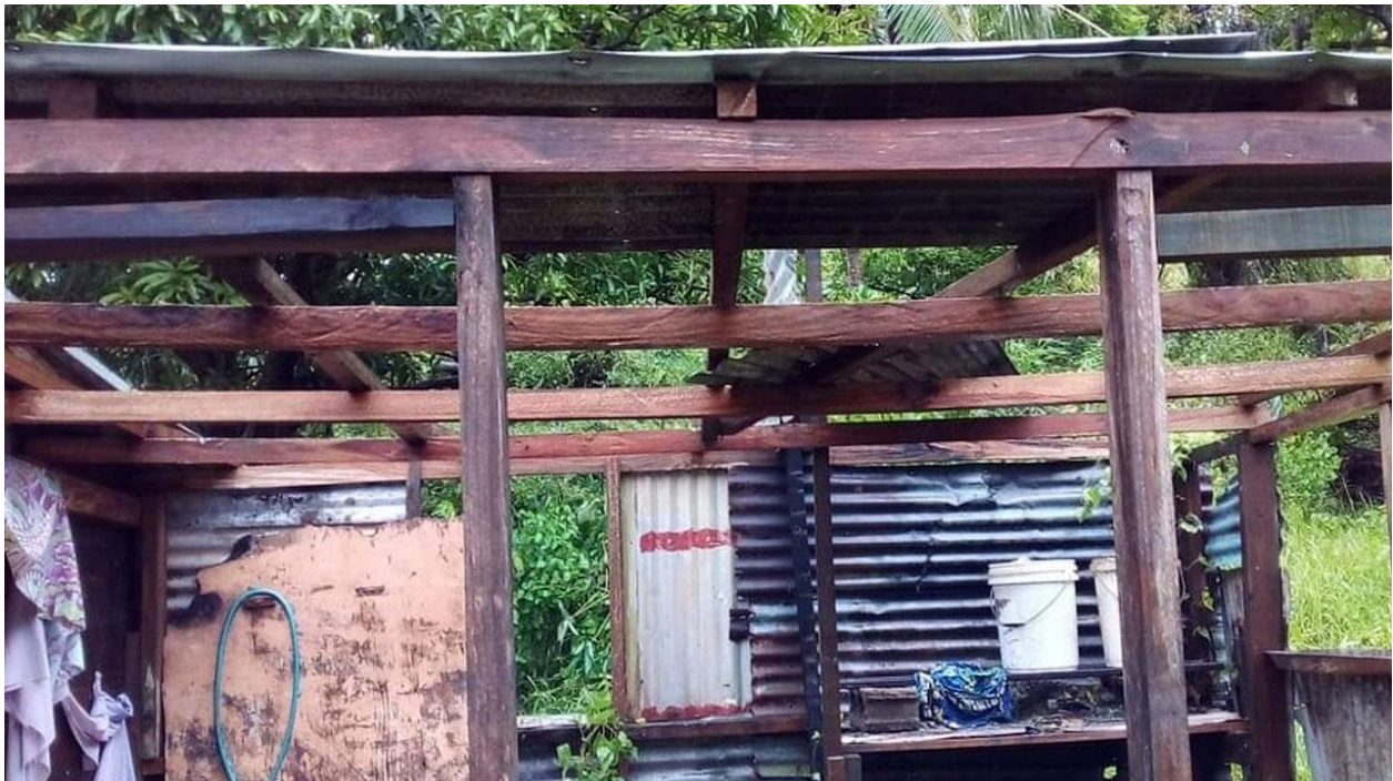
Damages to a house in Naqara, Kadavu due to TC Ana. Photo credit: TURAGA NI KORO, ISEI RAKADRUTI.
